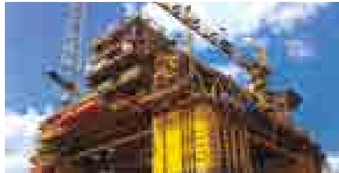
Gumusut-Kakap Semi-Submersible Floating Production System (FPS)
